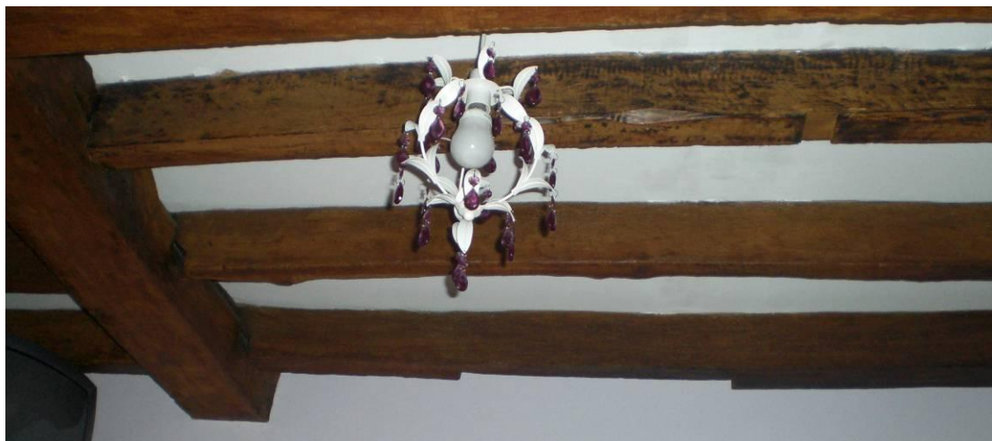
The joists in Bedroom 4. The one with the slot cut in it is probably Georgian - the others are later inserts.
